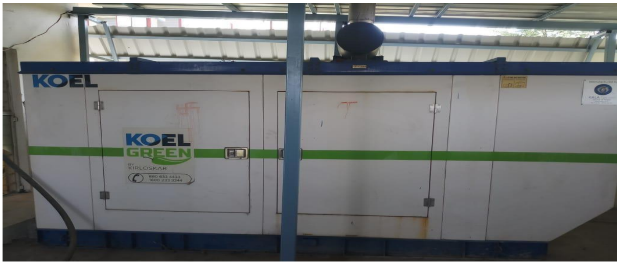
Figure 2.3 DG set in Power House
