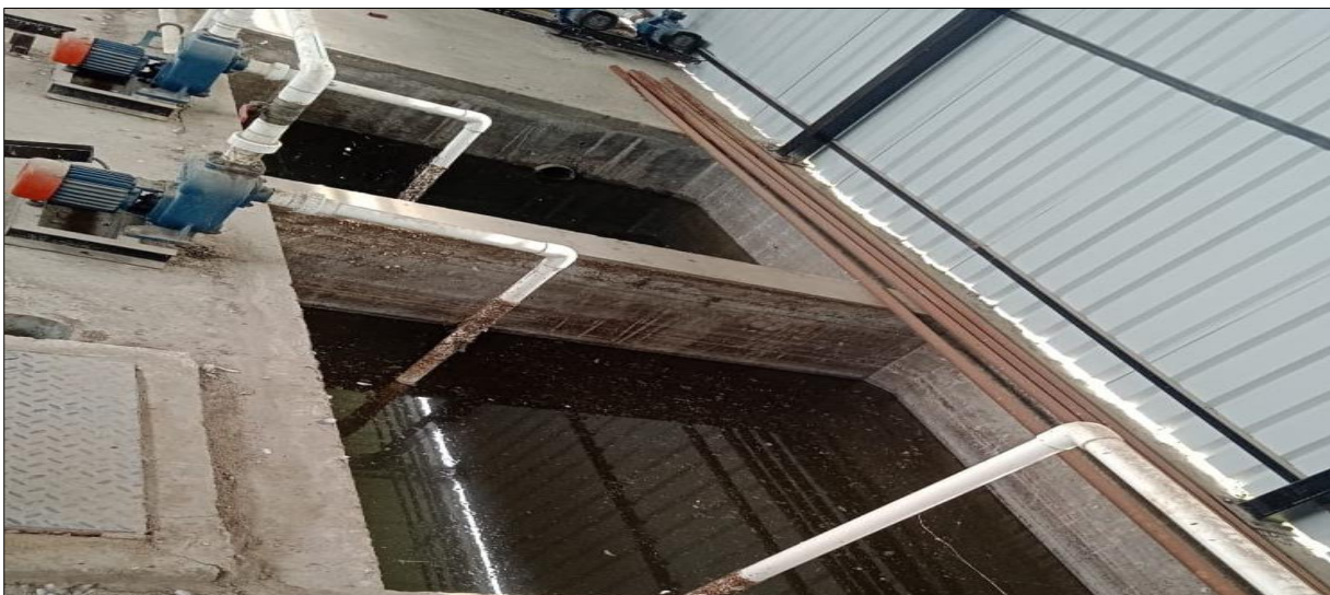
Figure: - 2.8 Sewage Treatment Plant in University
