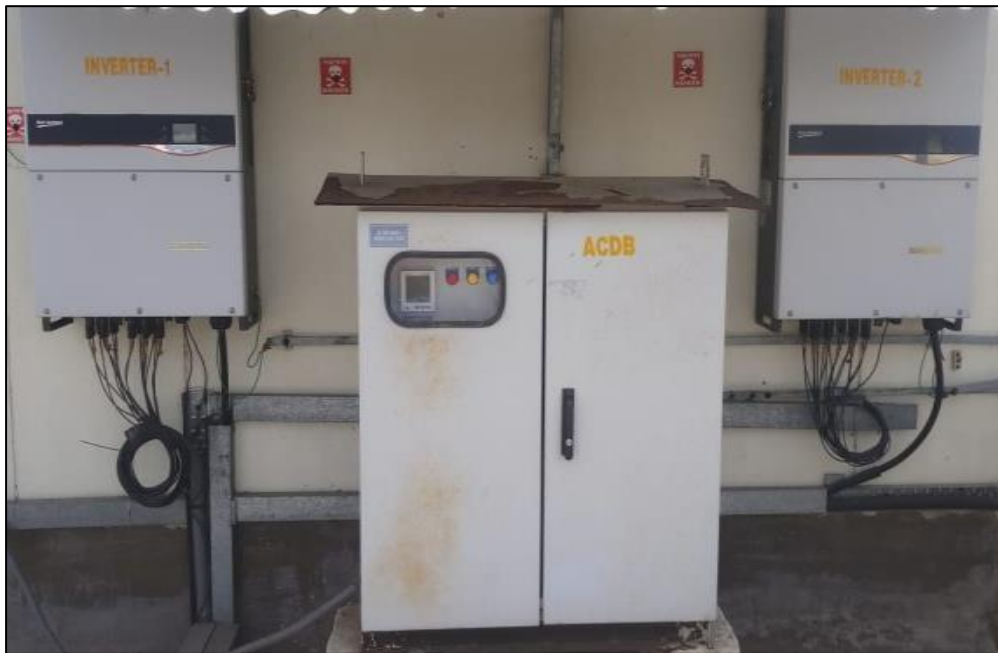
Figure 5.1: Solar Plant 100 KWp and Inverter System
