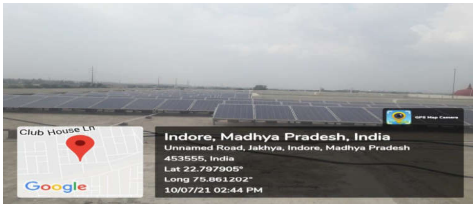
Figure 5: Details of Installed Solar Panels
