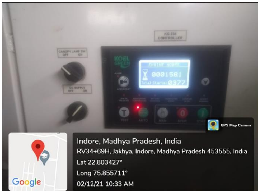
Figure.7: Relay Switch for Generator
