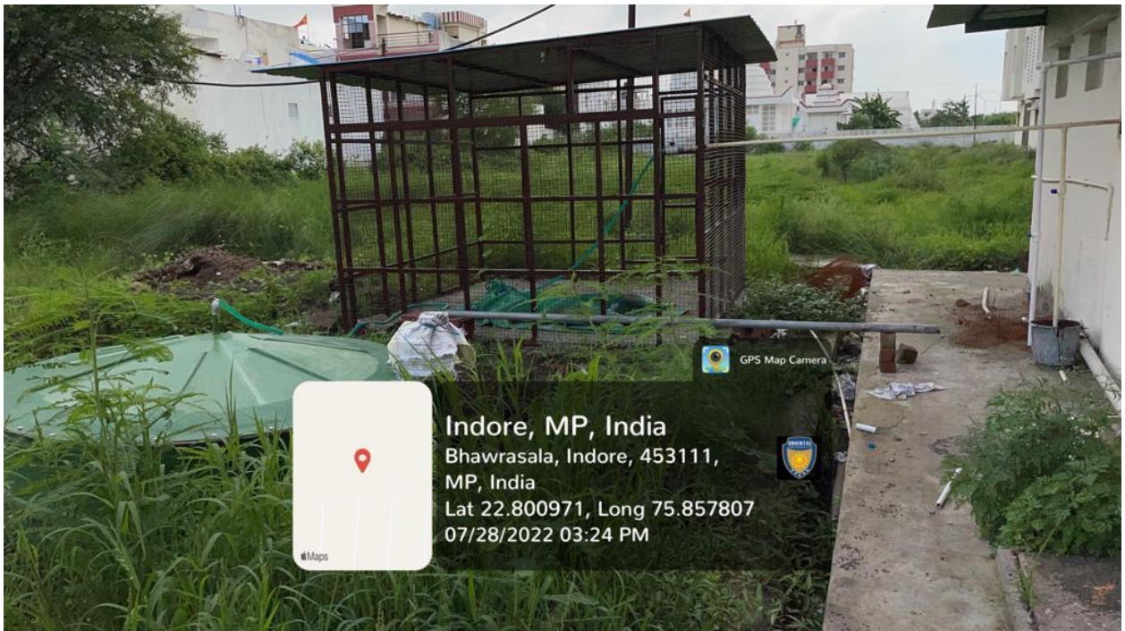
Figure.4: Biogas Plant installed at Oriental University Indore Campus
