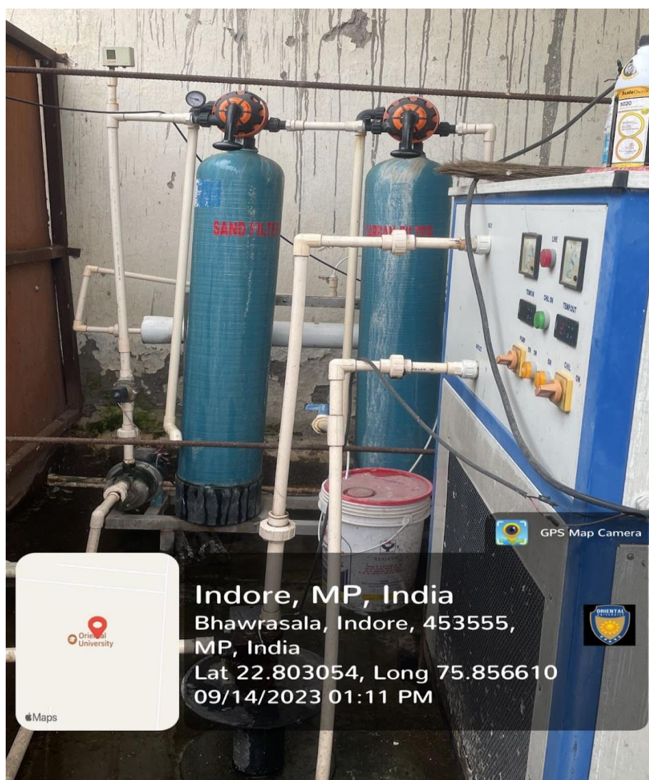
Figure.12: Reverse Osmosis (RO) Plant
