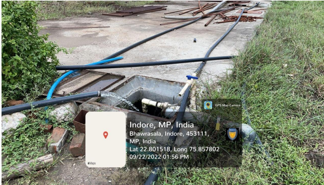
Figure.8: Geotag Photographs of storage tank in hostel areas
