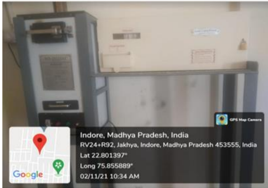
Figure.4 Sanitary Pad Incinerator
